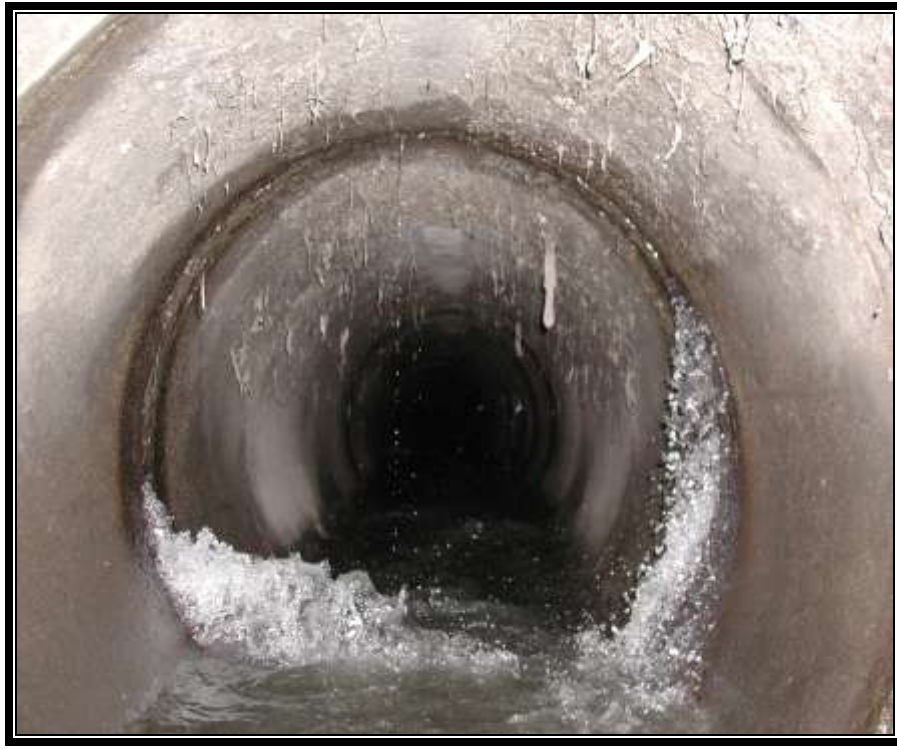
Figure 19: North Side Trunk Sewer immediately upstream of the Kelsey Creek Basin (003) CSO
